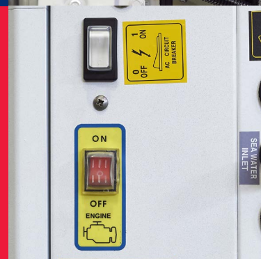
Main circuit breaker
